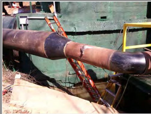
The screened flow from the creek is delivered by penstock .
