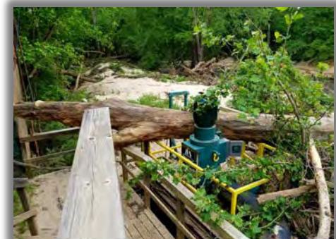
Once the water receded and logs removed, power was quickly back on.
