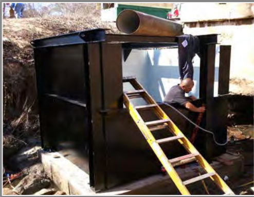
A splitter box is necessary for this site to handle the draft tube.
