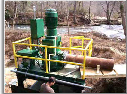
The pad, splitter box and platform support this entire system.
