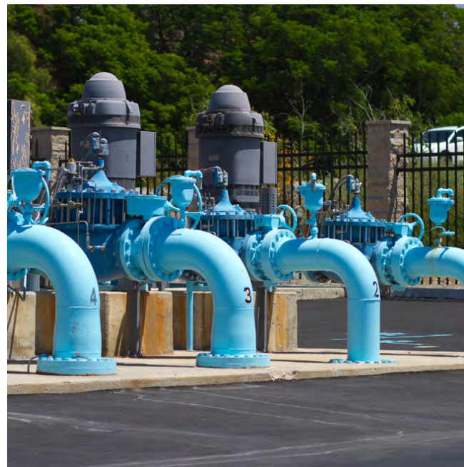
Pump Stations (Non-pressurized)
